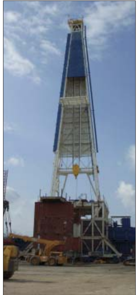
Parker Rig No. 262 mast sits fully raised in the construction yard at New Iberia, La. Clamps hold the substructure to rails that are attached to 40 driven pilings to counteract the moment created by raising the mast (Fig. 12). A similar rig up will occur at the Sakhalin drilling location. Photo courtesy of Parker Drilling Co.
